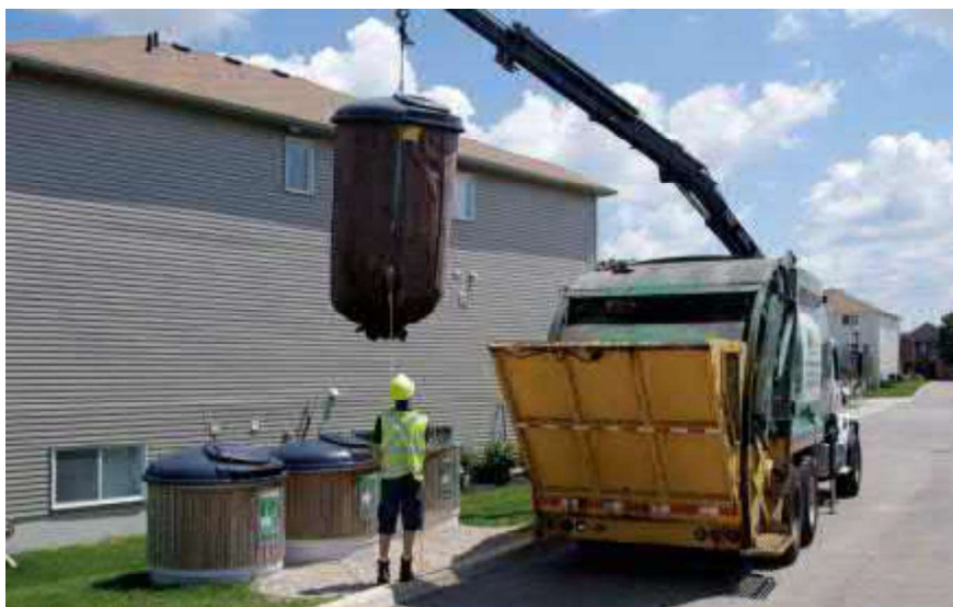
Figure 20: Waste collection for Molok underground bins
